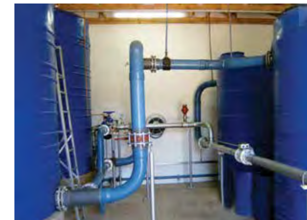
Above: View of part of treatment plant. Carbon filter on the left side and Contact tank on right side. Left: Installation of submersible pump with the recharge valve on top.
