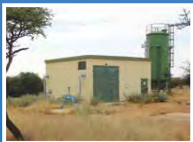
Managed aquifer recharge station
