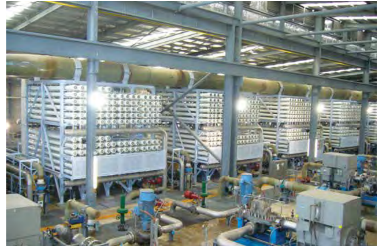
The Reverse Osmosis rack system
