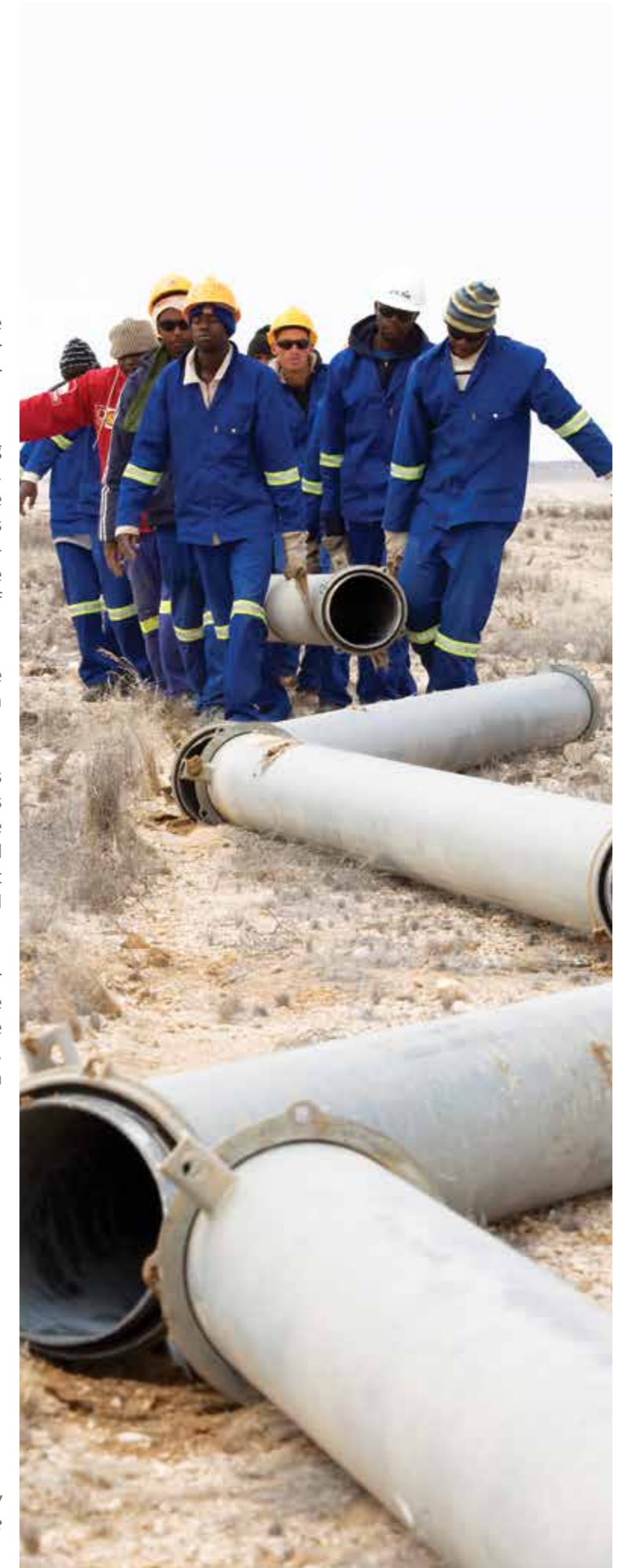
Construction of the 30 km temporary pipeline to Husab, which is now in place and already pumping water.
