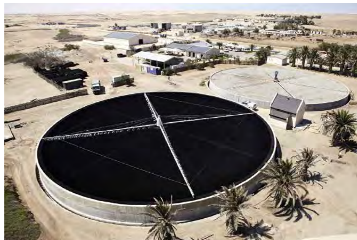
Part of upgrade of Walvis Bay's sewerage works that will significantly increase the plant's daily capacity from 2 mega litres to roughly 6.5 mega litres per day.
