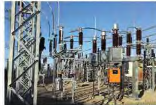
Auas Blick Sub-station
